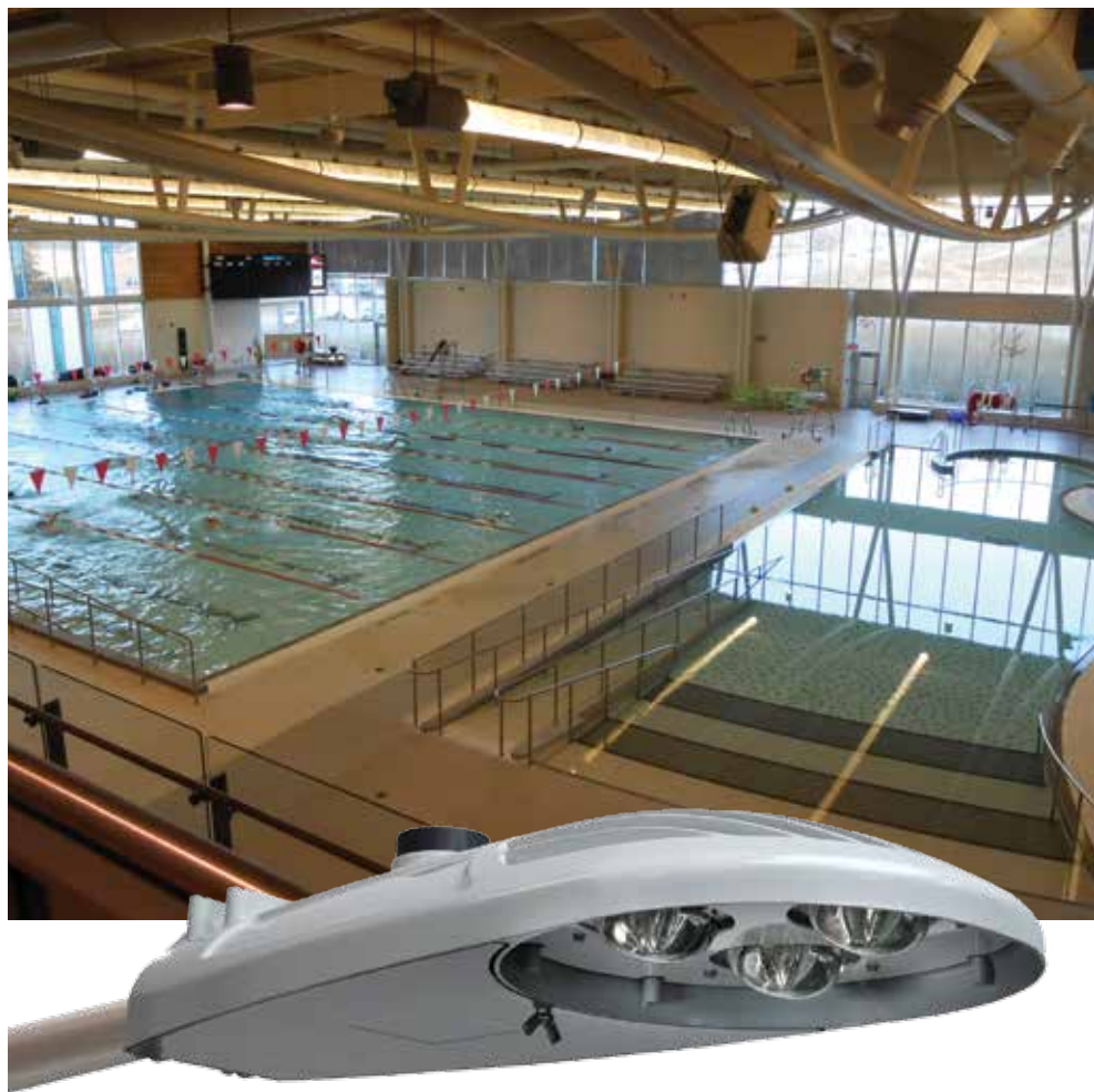
TOP: Honeywell expanded on Newmarket's Andover control and automation system that manages lighting and HVAC to allow for greater temperature control at numerous locations, including Gorham Pool.
